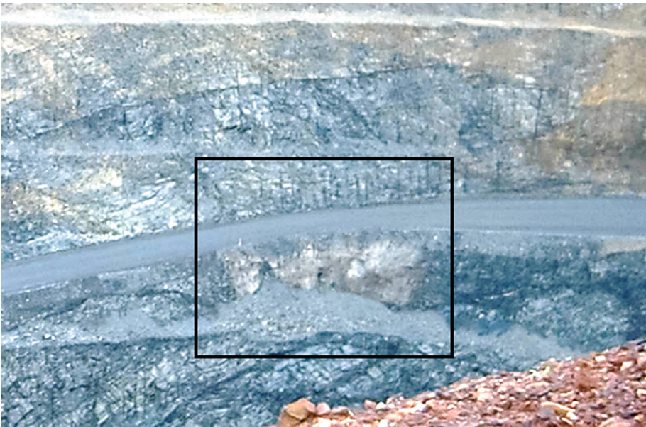
Fig. 4. Side-ramp failure (slabbing) at the open pit ramp, photo taken from the south in Feb. 2011
